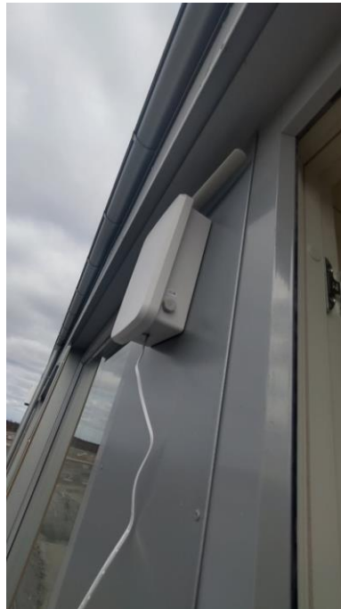
Wall-mounted outdoor sensor installation.
