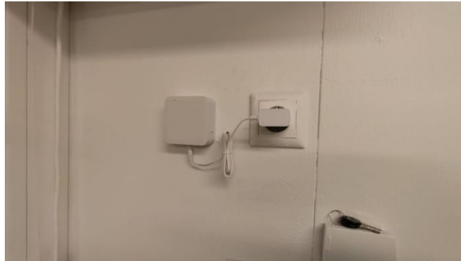
Wall-mounted installation in office area.
