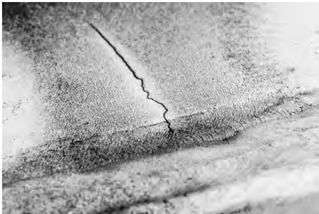
Fig. 18.5: Detection of a crack with magnetic flux inspection. The magnetic particles are black in this picture.
