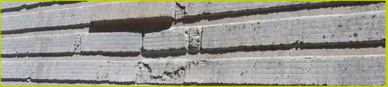
Spalling has occurred on edges of the liner plates because the gap between the liners was not properly filled with hardfacing wire.
