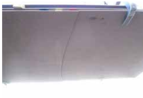
Example of a three-point lift with a crack as an result.
